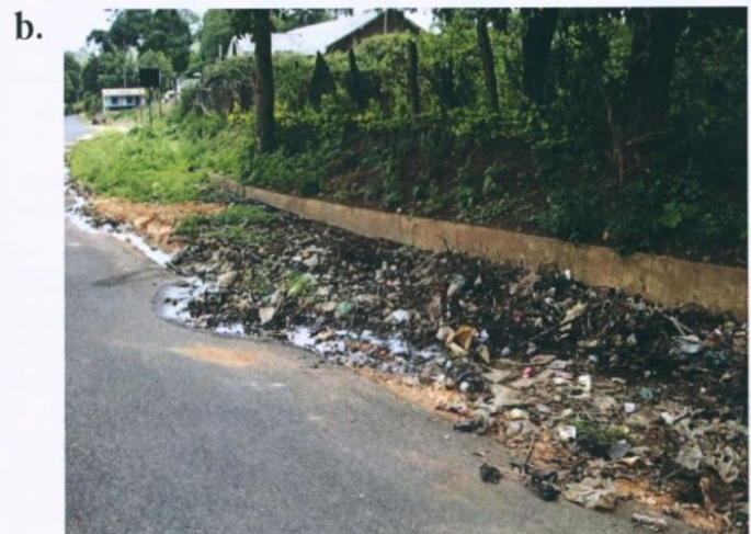
Figure 6: a. Picture of a clogged street gutter b. Picture of the rampant loitering and public defecation that lay on the side of the roads
