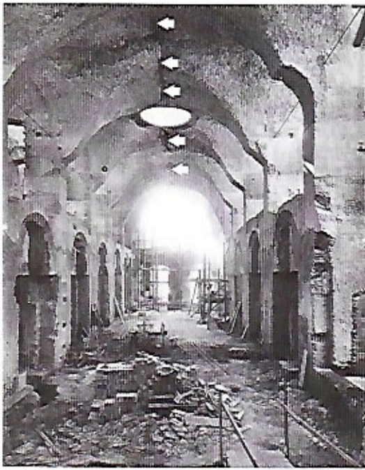
Figure 3- Great Hall Section with Damage
